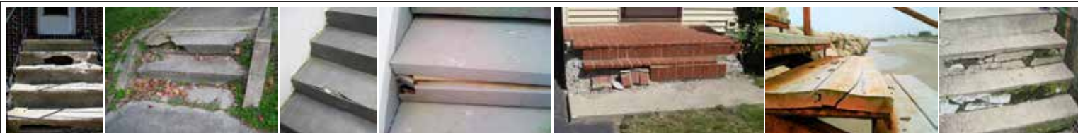
NON-Suitable Steps - Holes, Cracks, Broken Tiles, Missing Bricks, Severly Slanted
